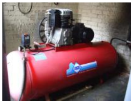
Reference: ATG-029 COMPRESSOR Year: 2004 Brand: AC DGM
