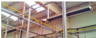
Reference: MOL-068 GAS HEATING RADIANT TUBE Year: . Brand: .
