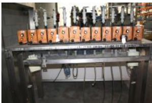
Reference: BPS-066 PUMP GROUP Year: . Brand: PROMINENT
