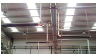
Reference: MOL-072 GAS HEATING RADIANT TUBE Year: . Brand: .
