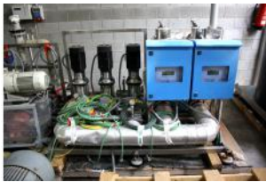
Reference: BPS-025 3 GROUP PUMPS WITH 2 GROUP UV ... Year: CRN 10-05 A-FGS-G-E-HQQE Brand: GRUNDFOS
