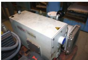
Reference: BPS-037 PUMP SUCTION Year: 1999 Brand: PFEIFFER
