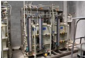
Reference: BPS-085 GROUP OF 3 TANKS ON STAINLESS ... Year: . Brand: .
