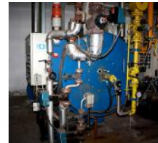
Reference: LUI-050 STEAM BOILER Year: 1998 Brand: BABCOCK WANSON
