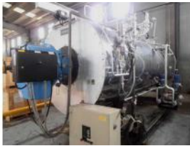
Reference: TIG-001 STEAM BOILER PIROTUBULAR HORIZONTAL Year: 2001 Brand: STEAMBLOC
