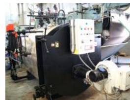
Reference: TPS-022 STEAM BOILER Year: 2001 Brand: VYC INDUSTRIAL
