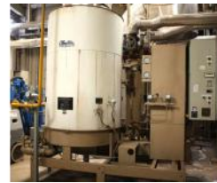
Reference: TIP-119 STEAM BOILER Year: 1994 Brand: CLAYTON
