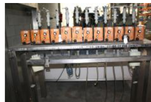
Reference: BPS-066 PUMP GROUP Year: . Brand: PROMINENT
