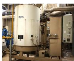
Reference: TIP-119 STEAM BOILER Year: 1994 Brand: CLAYTON
