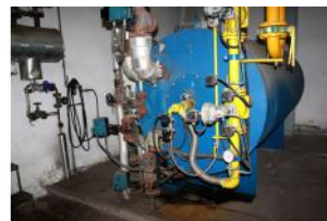
Reference: LUI-049 STEAM BOILER Year: 2000 Brand: BABCOCK WANSON
