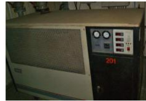
Reference: FSV-107 COMPRESSED AIR DRYER Year: 1992 Brand: CHAUMECA IBERICA
