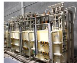
Reference: BPS-086 GROUP OF 4 TANKS ON STAINLESS ... Year: . Brand: .
