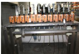
Reference: BPS-066 PUMP GROUP Year: . Brand: PROMINENT
