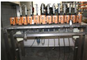
Reference: BPS-066 PUMP GROUP Year: . Brand: PROMINENT
