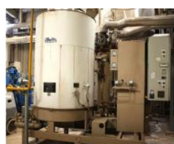
Reference: TIP-119 STEAM BOILER Year: 1994 Brand: CLAYTON
