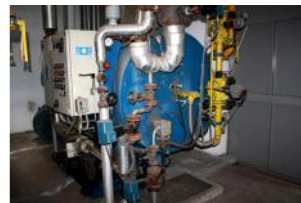
Reference: LUI-052 STEAM BOILER Year: 1998 Brand: BABCOCK WANSON
