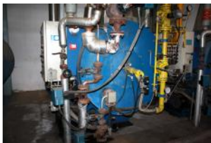
Reference: LUI-051 STEAM BOILER Year: 1998 Brand: BABCOCK WANSON
