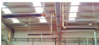
Reference: MOL-070 GAS HEATING RADIANT TUBE Year: . Brand: .
