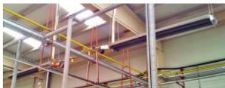
Reference: MOL-068 GAS HEATING RADIANT TUBE Year: . Brand: .
